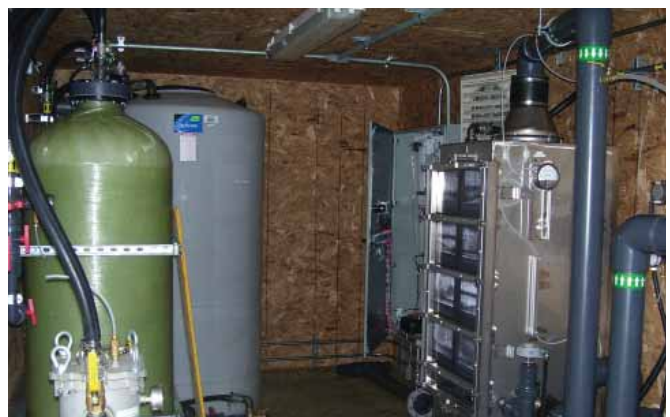
Interior photo of Northeast Area treatment system
