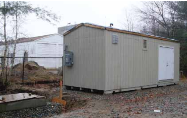
Exterior photo of Northeast Area treatment system
